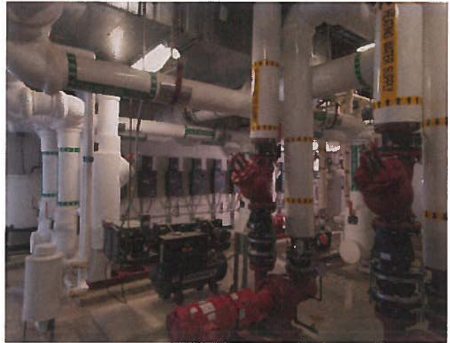
Water comes into the research facility from the Chesapeake Bay and gets conditioned (for purity and temperature) to be ideal for the cultivation of oysters. The temperature of the water must constantly be maintained within strict parameters, and the filtration pumps cannot fail.
