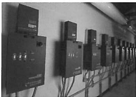
These MCH Series Variable Frequency Drives from AC Technology are controlling pumps, cooling towers and the building HVAC system in the research facility.
